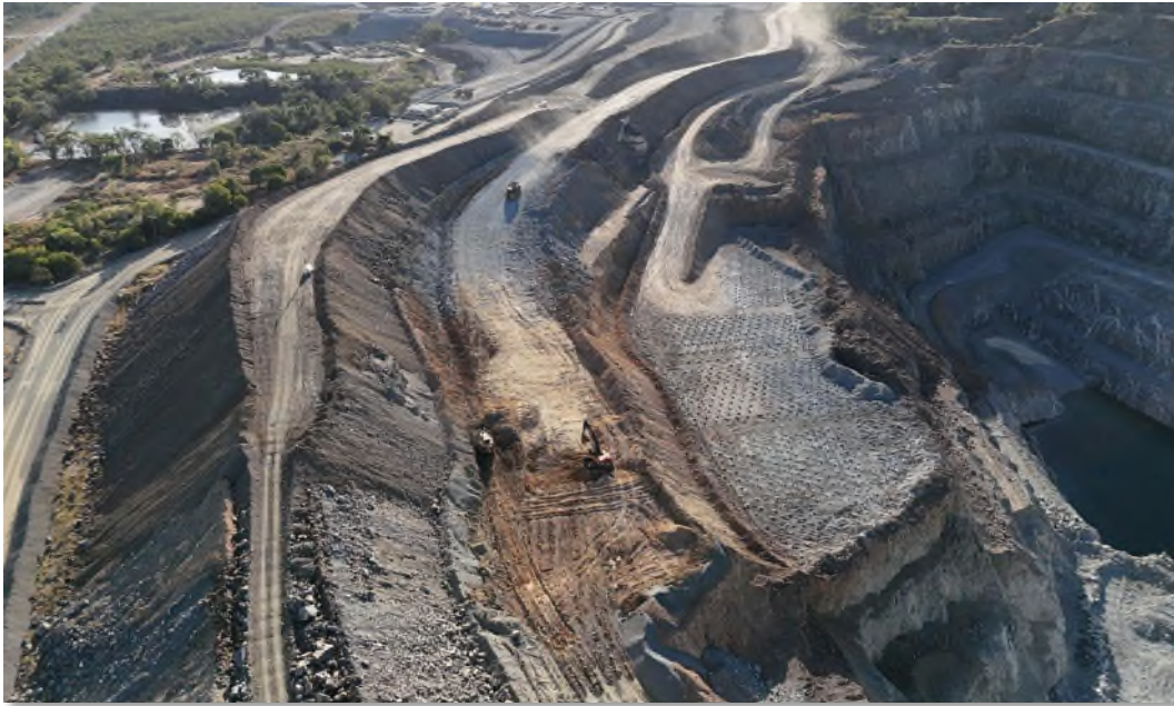
Picture above: Stripping activities progressing in the South side of the open pit where the old processing plant use to once stand.
