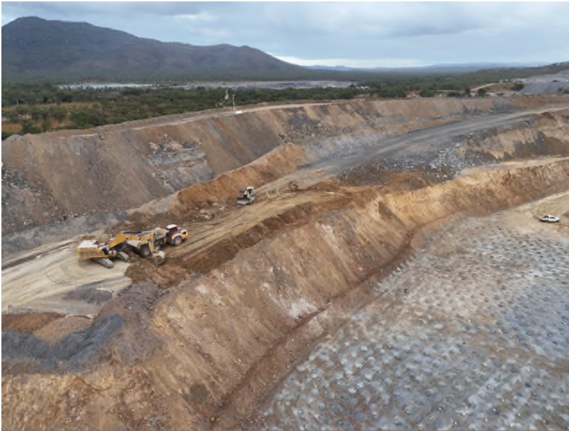
Picture above: Mining operations progressing in the Southern area of the pit
