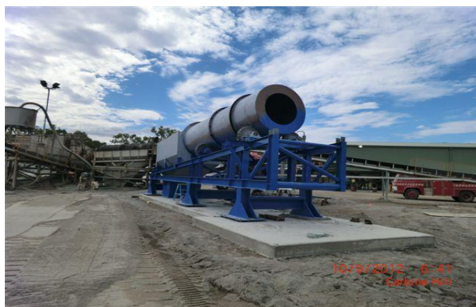
New front end scrubber
