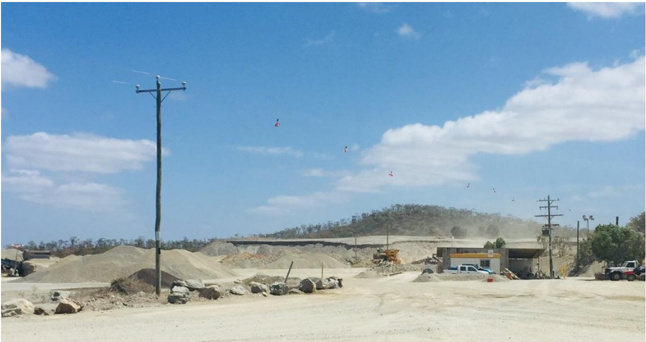
Figure 9: 22kV Power Lines at the Crushing and Screening Plant
